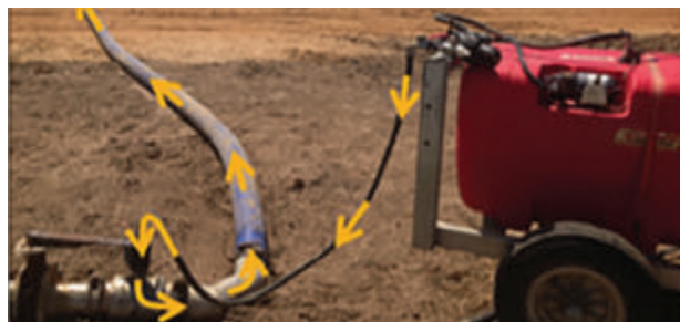
Figure 1: An example of a TERVIGO application system, here the injection solution is mixed in the red supply tank then injected into the pressurised mainline using a 12 volt pump.
